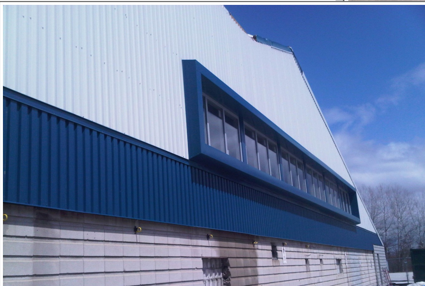
The new façade, with its energy efficient glazing is complete and the tarp has been removed.
