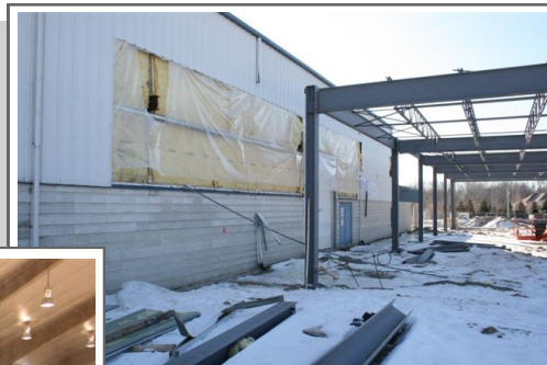
Steel beams for west end community hall being tied into existing building structure..
