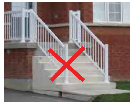
Precast stairs (not permitted)
