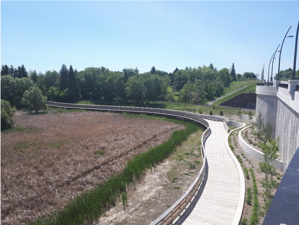
Nokiidaa Trail Boardwalk System through Wetland – East Gwillimbury Partnership Project with York Region and Lake Simcoe Region Conservation Authority
